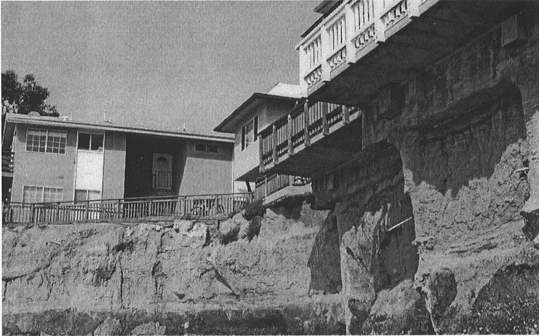
Figure 5. Undercut apartments on the cliff in the Isla Vista area of Santa Barbara County.
