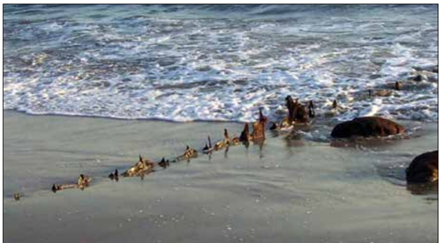
Figure 16. Dilapidated sheet-pile groins left hazards along the shoreline at Las Tunas Beach, Los Angeles County, California
