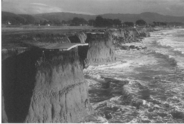
Figure 16. Severe bluff erosion south of the Half Moon Bay breakwater led to loss of oceanfront road and sewer line.
