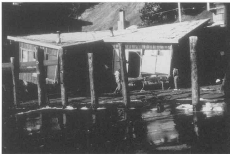
Figure 15. Severe El Niño related beach scour in the winter of 1982-83 at Rio Del Mar led to undermining of piling foundations and collapse of beach level homes.
